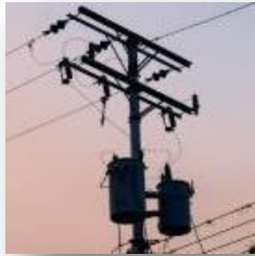
Close proximity to 3-phase powerlines with available capacity
