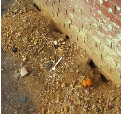
Norway rat burrows may be found singly or in groups, such as these along a school foundation wall. (Photo L. Pinto)
