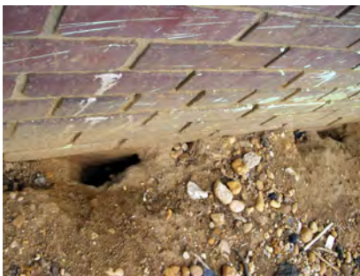
Around structures, the preferred sites for Norway rat burrows are under concrete slabs and along foundation walls. (Photo L. Pinto)
