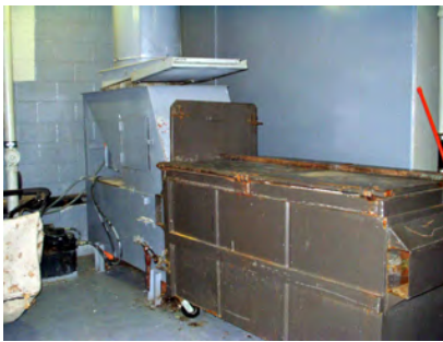
Rats or mice can live inside the block walls around a trash chute many floors up, and come down at night to feed in and around the compactor. (Photo L. Pinto)
