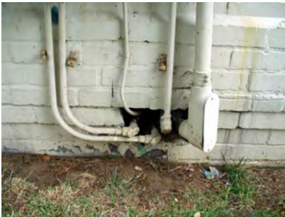
Utility conduits that provide entry points into a building include electrical lines or gas lines, TV cable or telephone lines, openings around water pipes, outdoor spigots, and water discharge lines from sump pumps. (Photo L. Pinto)
