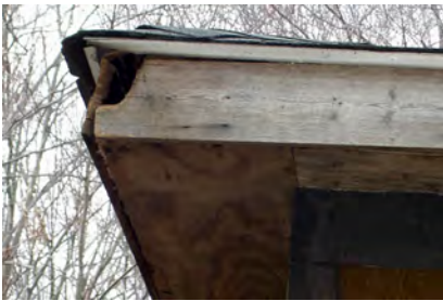
Seal, screen, repair or otherwise rodent-proof openings on and around the roof that can let rodents into the building. (Photo L. Pinto)
